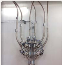
Multi-line for the feeding of the weighed cyclone; allows the production of the pre-mix during the transfer phase
